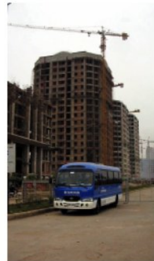
The building in the foreground was the first in Vietnam to have the Sanishute™ System installed. The system is now being installed in the next five buildings in the background.
