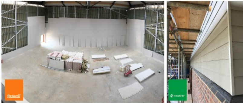
Joint fermacell (interior) and James Hardie (exterior) project "Bunn Leisure, White Horse Building" in UK
